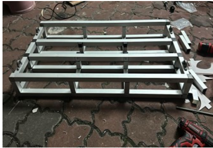
Figure 6 Micro Hydropower Frame
